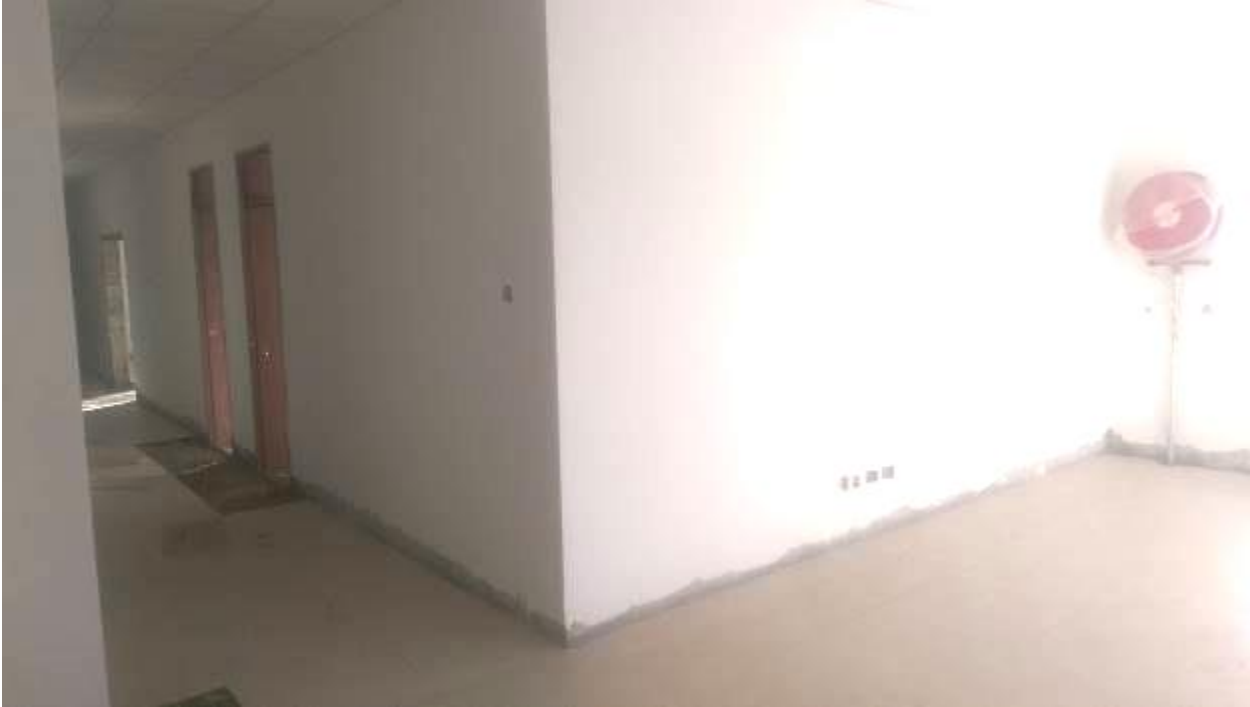
Figure 9: Office Finishes. Floor Tiling, Partition walls with Door Frames and Ceiling Installation
