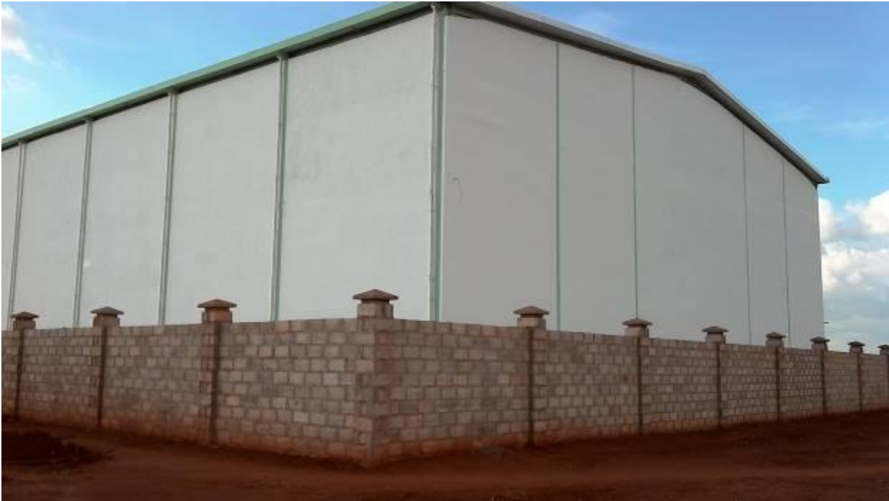
Figure4: Completion of External Wall Plastering and wall finishing with 1 st Coat of paint.
